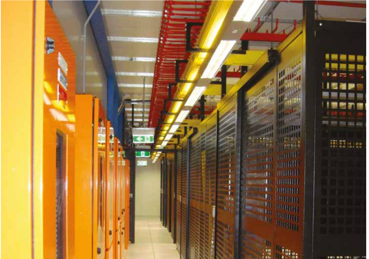
Equinix Data Centre SY3 Australia
